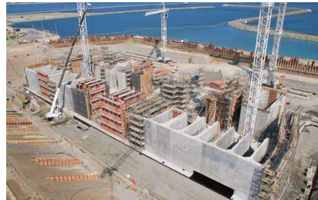
MAJIS SEAWATER INTAKE AND PUMPING STATION Sohar, Oman
